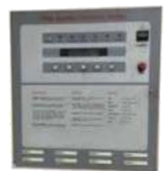
FIRE ALARM PANNEL
