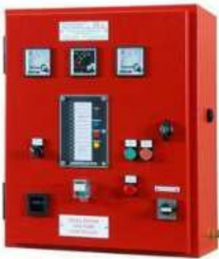
CONTROL PANEL FOR FIRE SYSTEM
